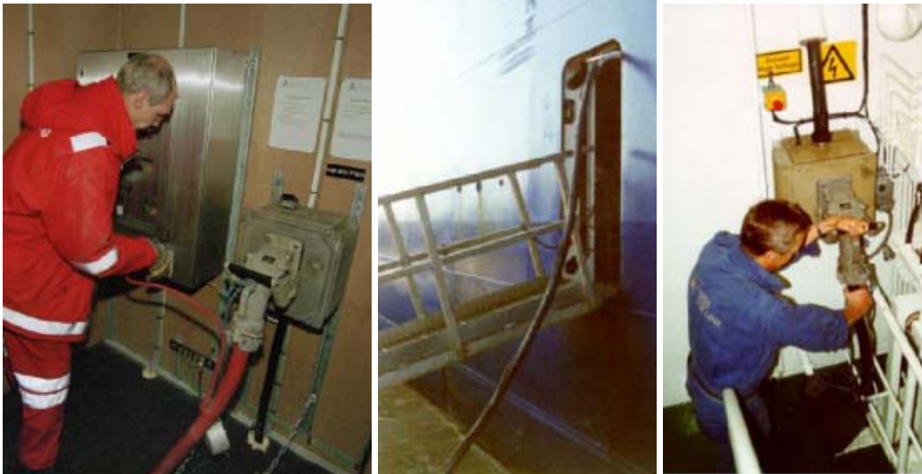
Figure 4 Connection practicalities (Photos: Port of Gothenburg)
